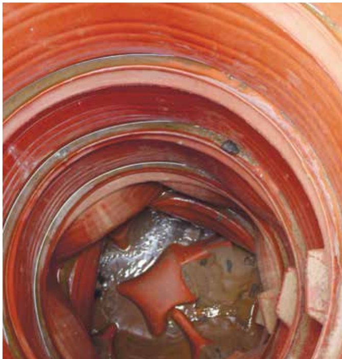
Pic. 1. Deformation of base and shaft of the manhole made using rotational moulding method.
