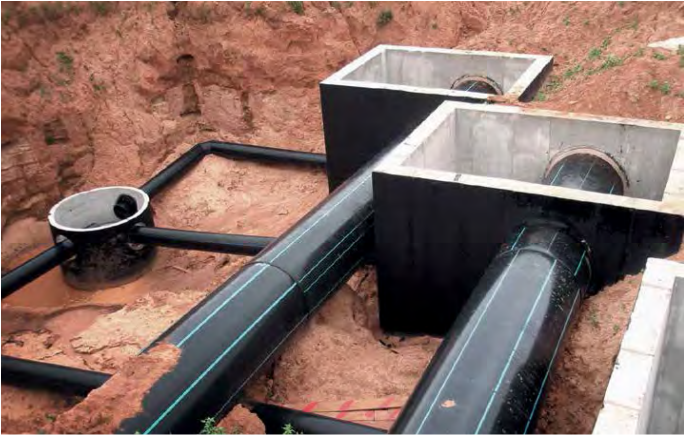
Pic. 1. Chambers and drainage wells.
