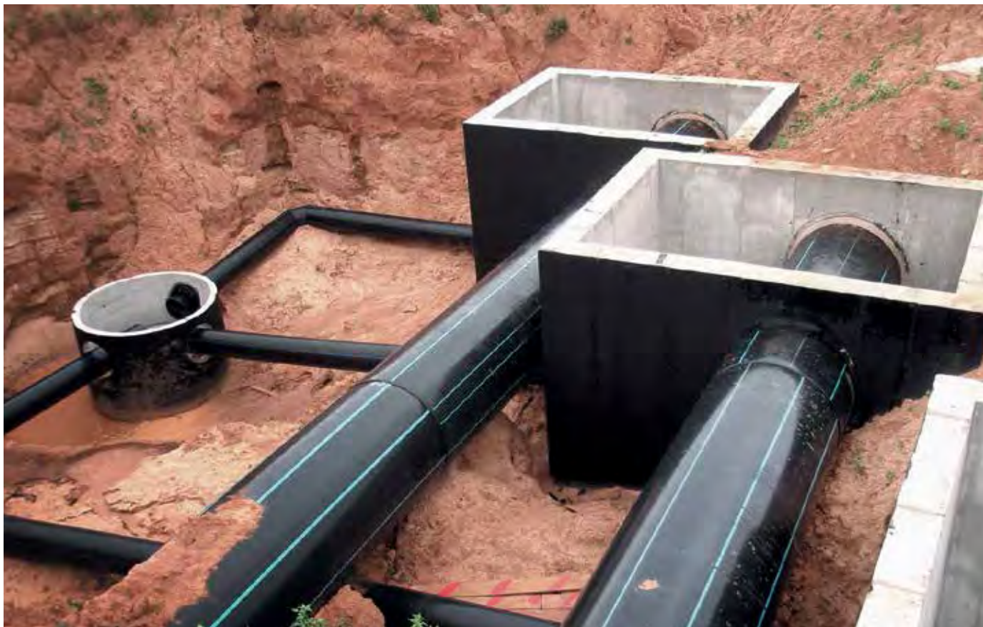
Pic. 1. Chambers and drainage wells.
